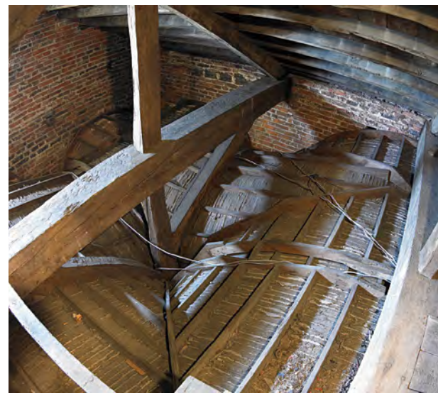
From above it's clear that this vaulted ceiling is formed from wooden lathes and plaster
