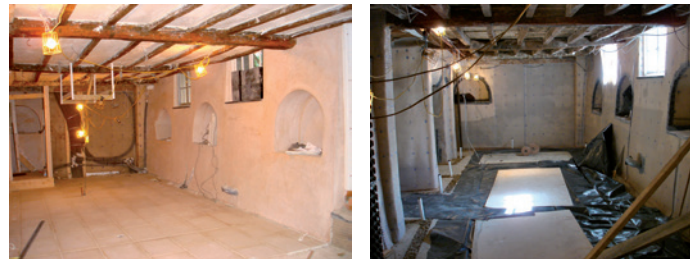
Platon Plaster Mesh was used to waterproof walls which had to be plastered directly including the small archways in the kitchen.
