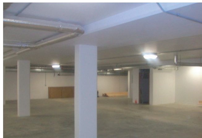
Triton products were used in the production of 450m 2 of watertight concrete used to construct the basement car park
